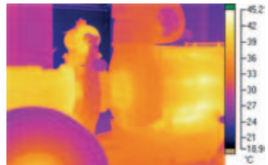
Fig. 8: Thermogram of the drive
